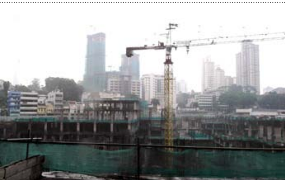
Abandoned Plaza Rakyat in Jalan Pudu effected DBKL - Plaza Rakyat Sdn.Bhd joint-venture
